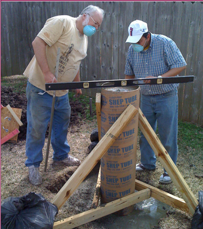
Tim Cowden and Anjal Sharma check the level of Anjal's backyard, concrete astro-imaging pier during construction.
